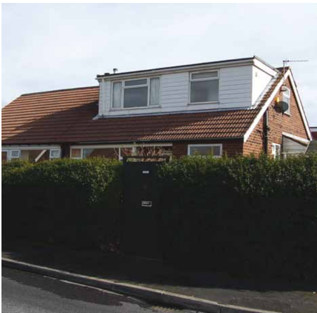
This dormer is located in a prominent position on the property and the use of materials which do not match or complement the roofscape makes it a very stark addition.
