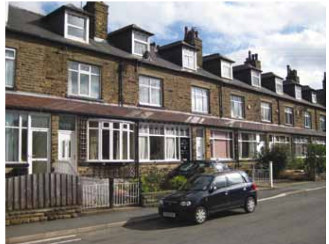
These dormers are small additions which are well positioned in the roofscape and do not cramp the chimneys. They sit above the existing first floor windows, use appropriate materials and are suitable to the age and style of the house.
